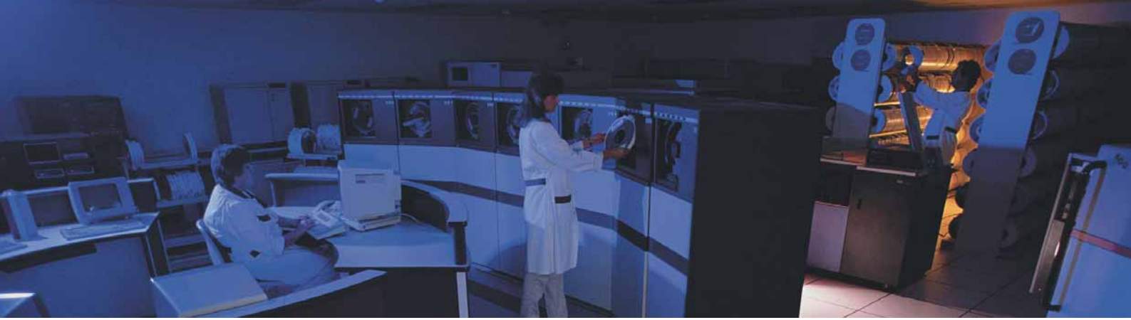
Data centre: Security application
